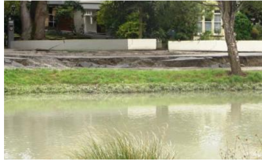
Figure 1. River bank slump.
